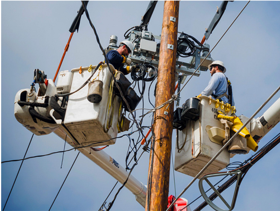
PP&L Electric Utilities Company will place wooden matting around utility poles near Claremont Gate and Bldg. 870 beginning at 8 a.m. tomorrow, Aug. 14. PP&L's activities will minimally impact traffic through the gate. (Photo by PP&L)
