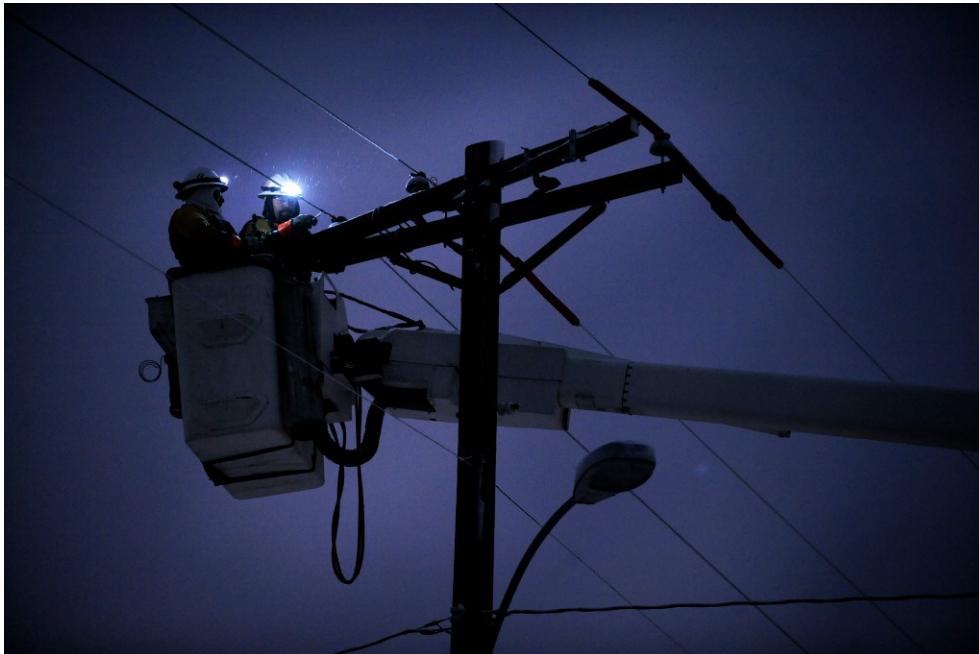
A power outage due to a transformer malfunction has caused organizations at 632 Wright Ave to close and relocate.
